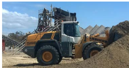
Pictured: L 566 Wheel Loader on site at Coast to Coast Dredging's sand pit in QLD.
